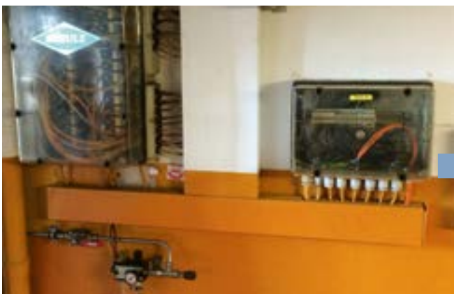
Before: Plastic cabinet with obsolete valve technology, porous hoses and plastic cable ducts
