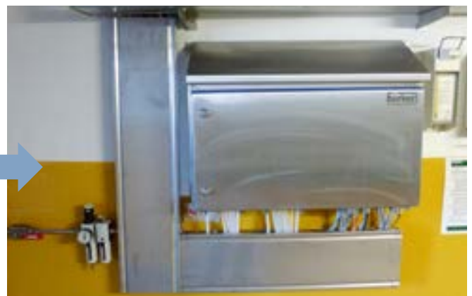
After: Stainless steel cabinet featuring hygienic design incorporating the latest valve technology, new piping and stainless steel mesh cable trays with cover
